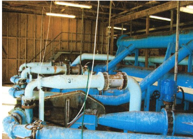
Figure 4-4: Manuwai Pump Station at Kerikeri
