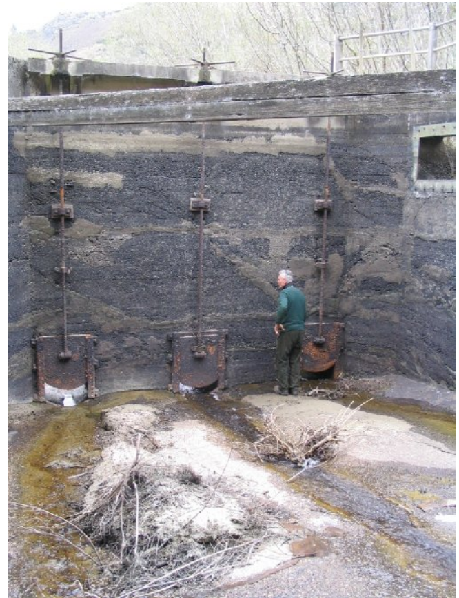
Figure 2: De-silter at the outlet of Tunnel No. 1
