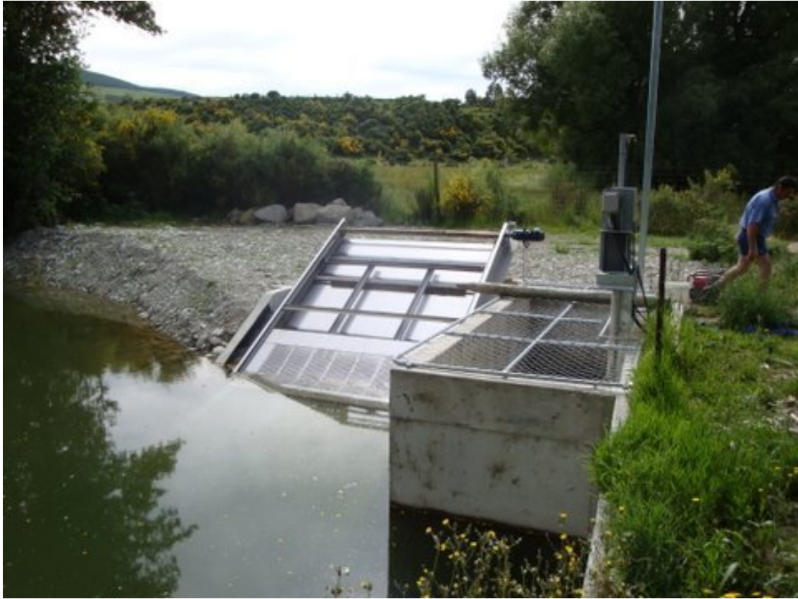
Figure 6-1: Intake of Kakahu Irrigation Scheme in South Canterbury
