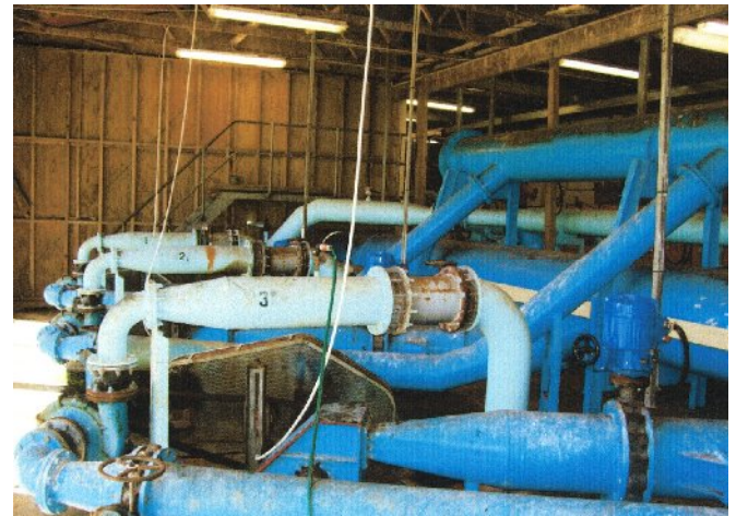
Figure 2: Manuawai Pump Station
