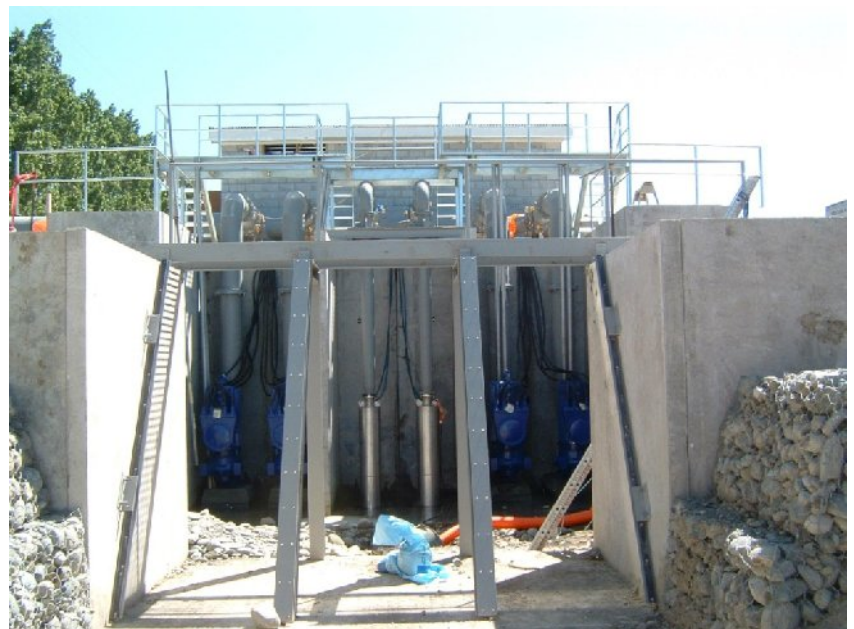
Figure 4: Main intake pump station
